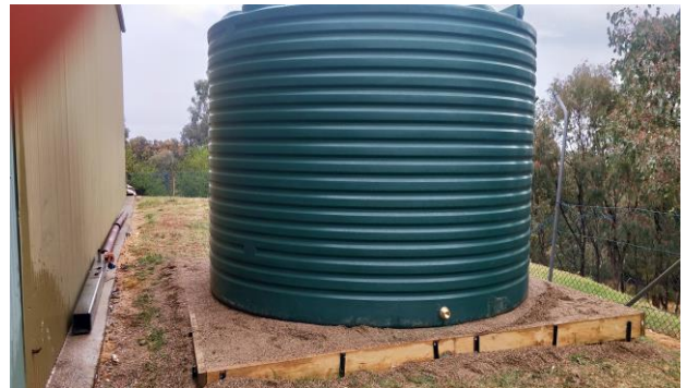
New Water Tank
